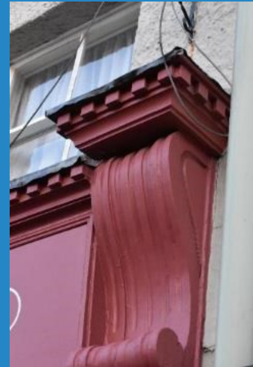
Figure 28 A narrow cornice with dentils on an early 20 th century shopfront, Oswald Road.
